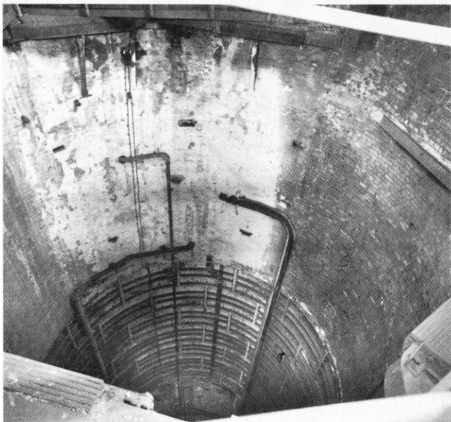
Lift Shaft - Note the lower lift landing at the bottom of shaft. Photo by Nick Catford
